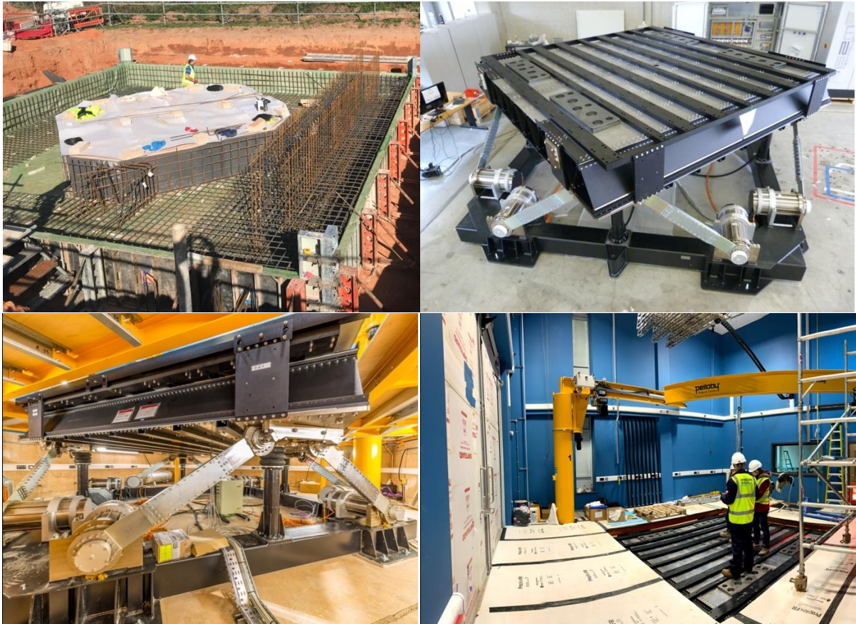
Motion platform: clockwise from top left: 50 tonne concrete foundation; factory acceptance at E2M, Amsterdam; installation in Exeter; view from basement level
